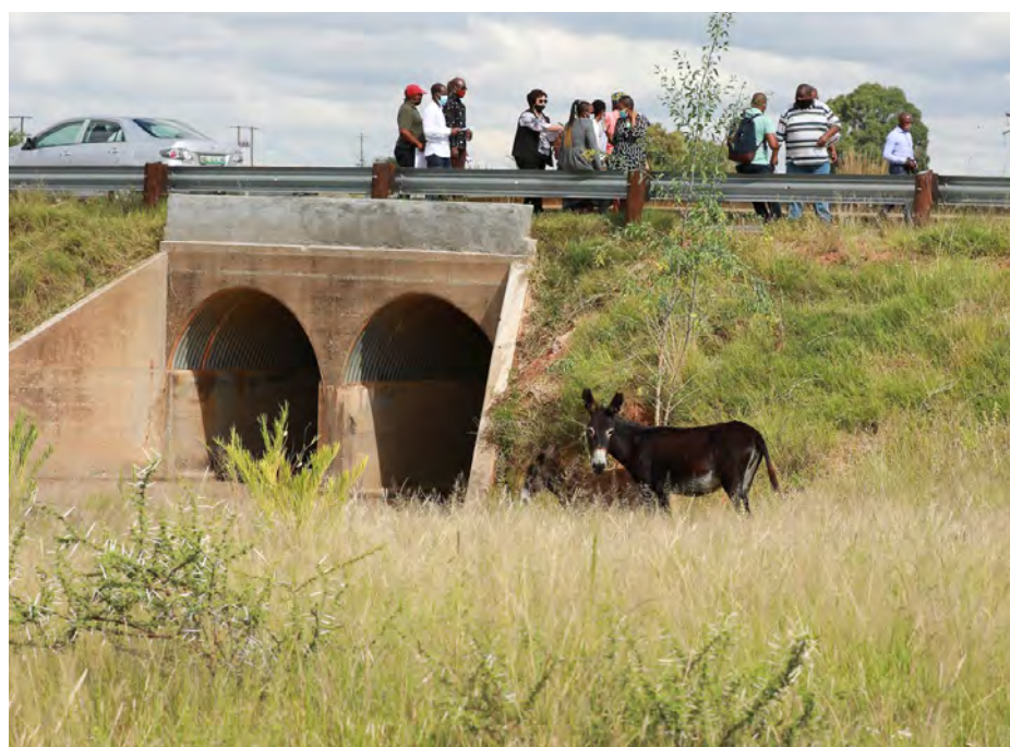
SMOOTH RIDE: The NCOP delegation inspected the reconstruction of the road after residents complained that potholes were making their life a misery.
