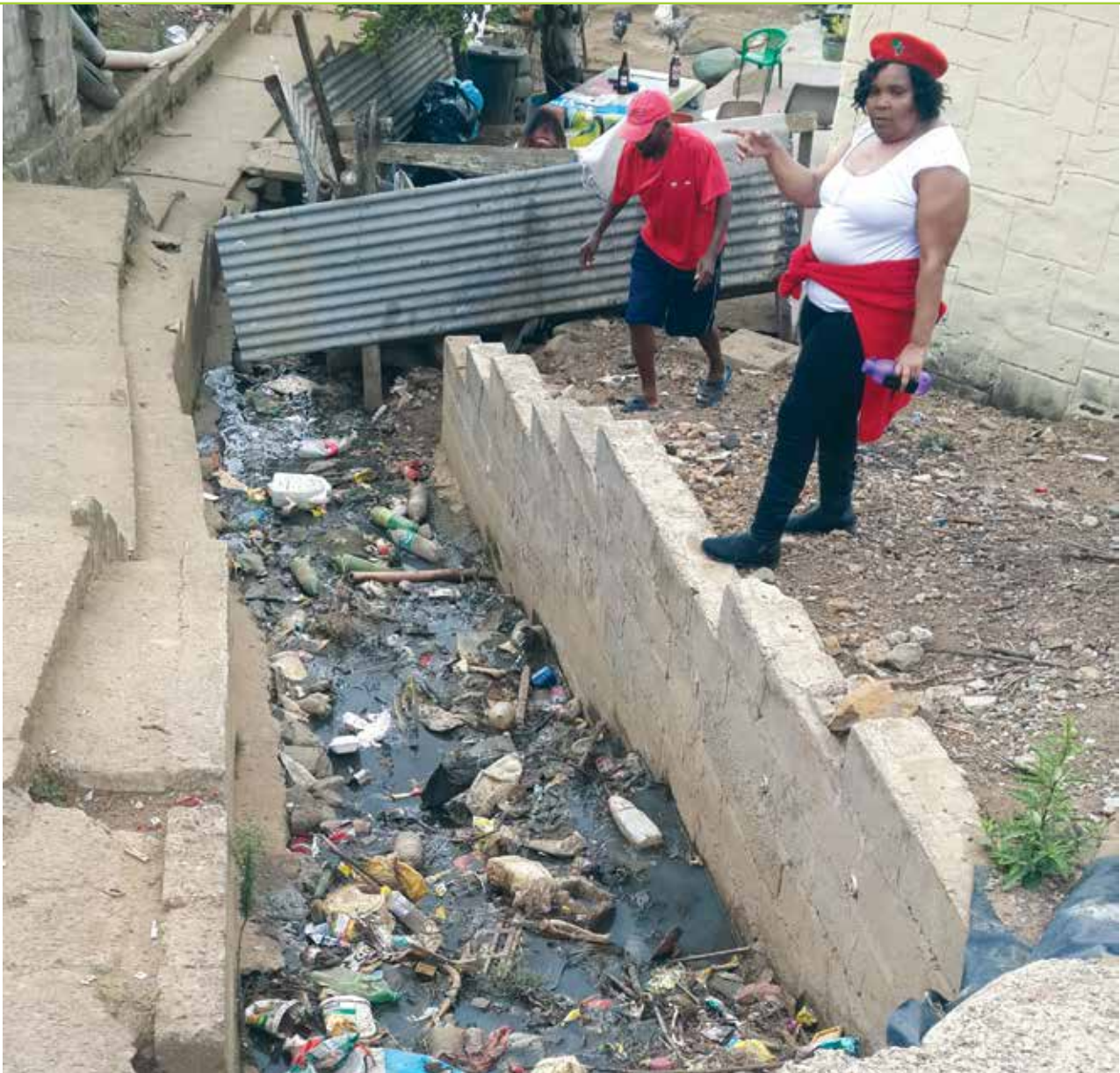
HEALTH HAZARD: EFF MP Ms Sibongile Khawula inspects one of the dirty canals that the residents of Inanda in KwaZulu-Natal blame for the rats that terrorise the neighbourhood.
