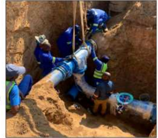
A pipeline upgrade to improve water supply in KwaNyuswa is at an advanced stage.
