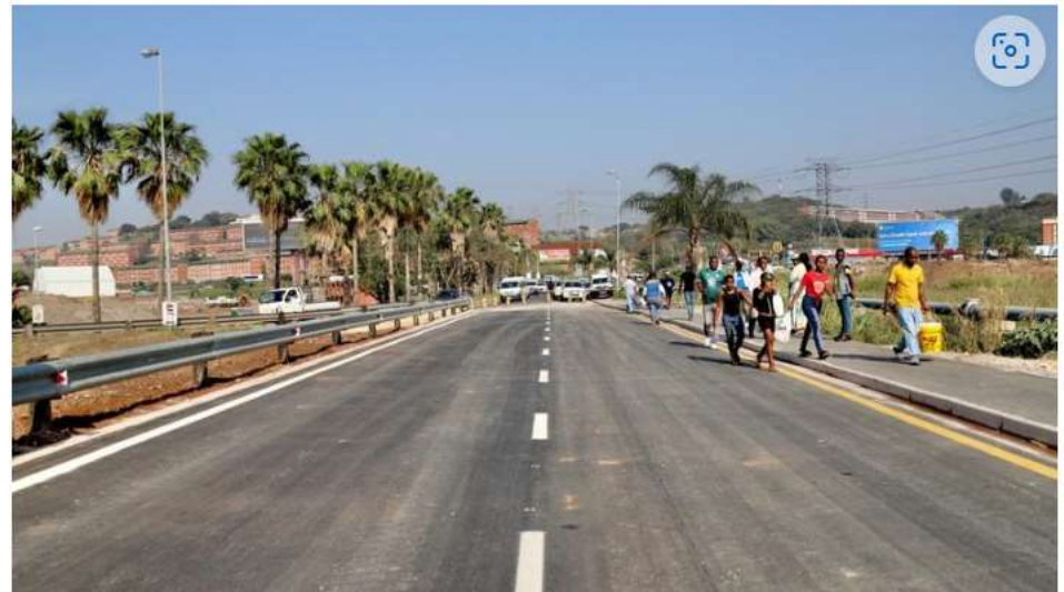
One of the busiest roads which were damaged in uMlazi during April floods have been repaired. Picture: Supplied
