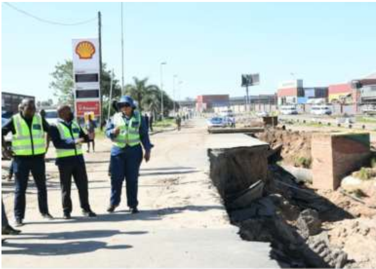
The extent of the damage following the April floods. File Picture
