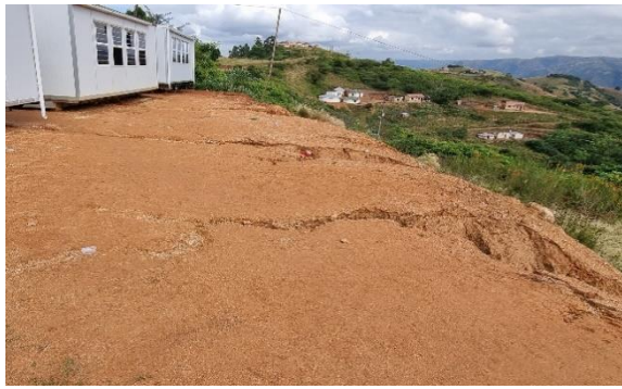
Poor drainage and erosion
