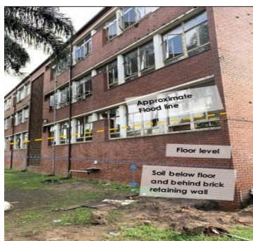
School classrooms structurally unsafe for use
